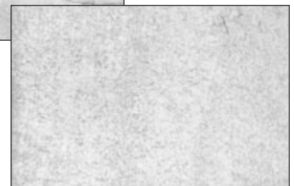
Reduced plastic shrinkage cracks with synthetic fibers
